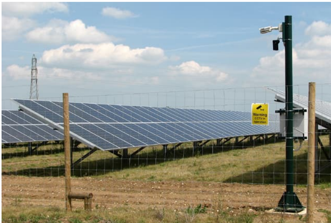
Plate 3-4: Example of Security Fencing and Monitoring Cameras
