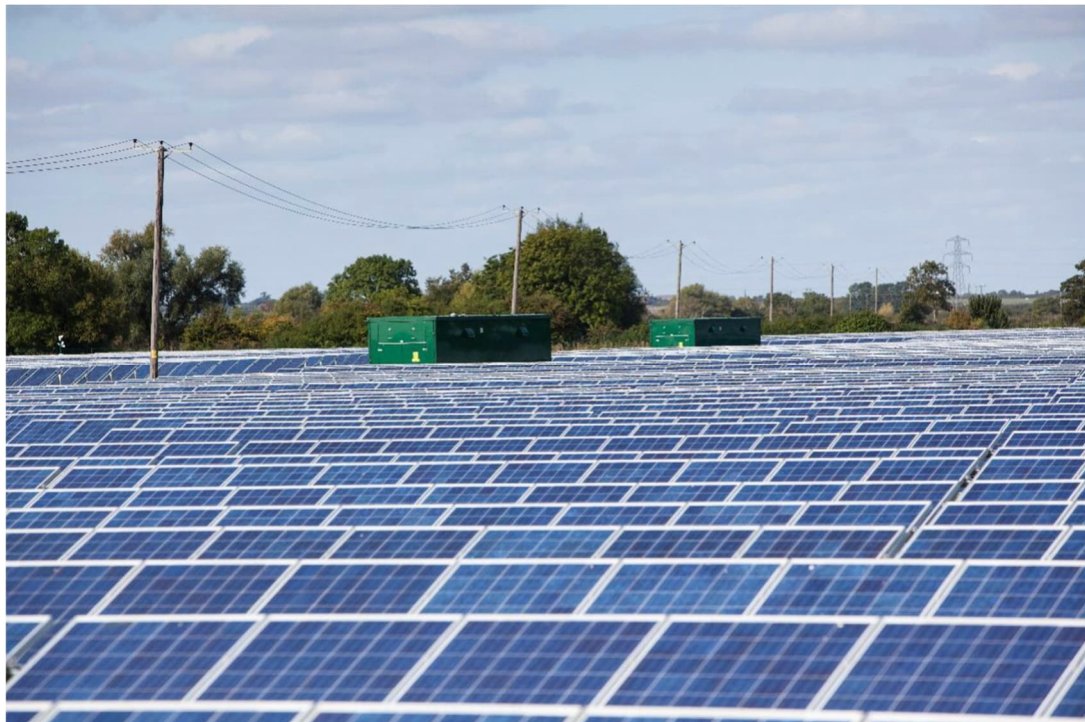
Plate 3-3: Example of Electrical Infrastructure Containers Located Within a Solar Array Substations and Control Buildings
